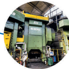
2009 Installation of the 6300 Ton press
